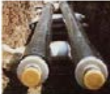
Figure 2 District Heating Network Pipes (size will vary)
